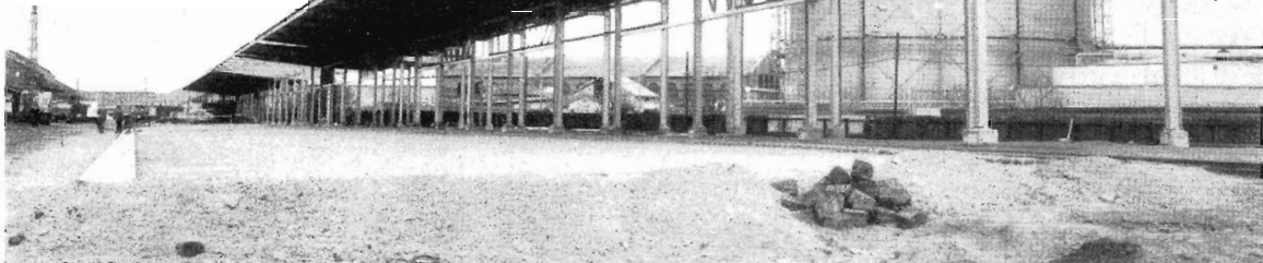
New No. 5 Shed is 1,070 ft. long, and wide enough to cover both road vehicle and rail wagon. The full length of the shed was brought into use on July 25, and the work previously done at Nos. 9 and 10 roads, Cowper Street, was transferred to it.
