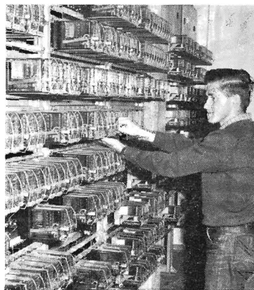
Signal Maintenance Fitter G. Wakefield removes a relay from the rack in the relay room. Relays are of the latest miniature type, needing much less mounting space.
