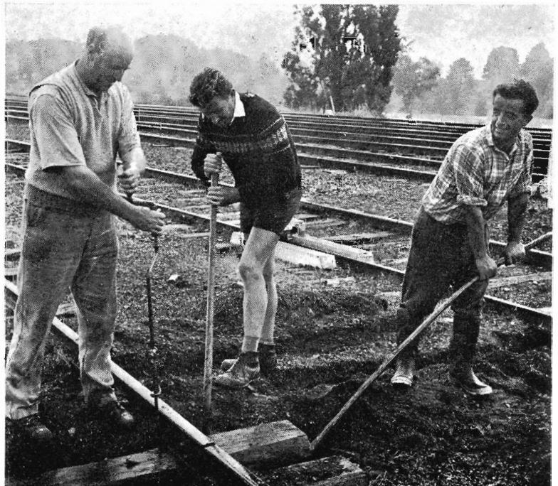
(From left) Repairer H. Benton, Ganger J. Walsh and Repairer G. Bruni replace sleepers in Malmsbury siding.
