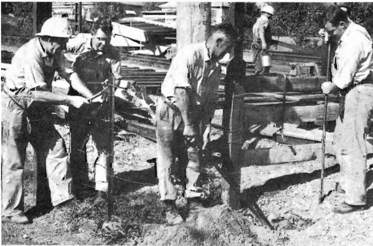
Members of Special Works gang are constructing a crib crossing in place of the footbridge. The crossing will later be replaced by a pedestrian subway.
