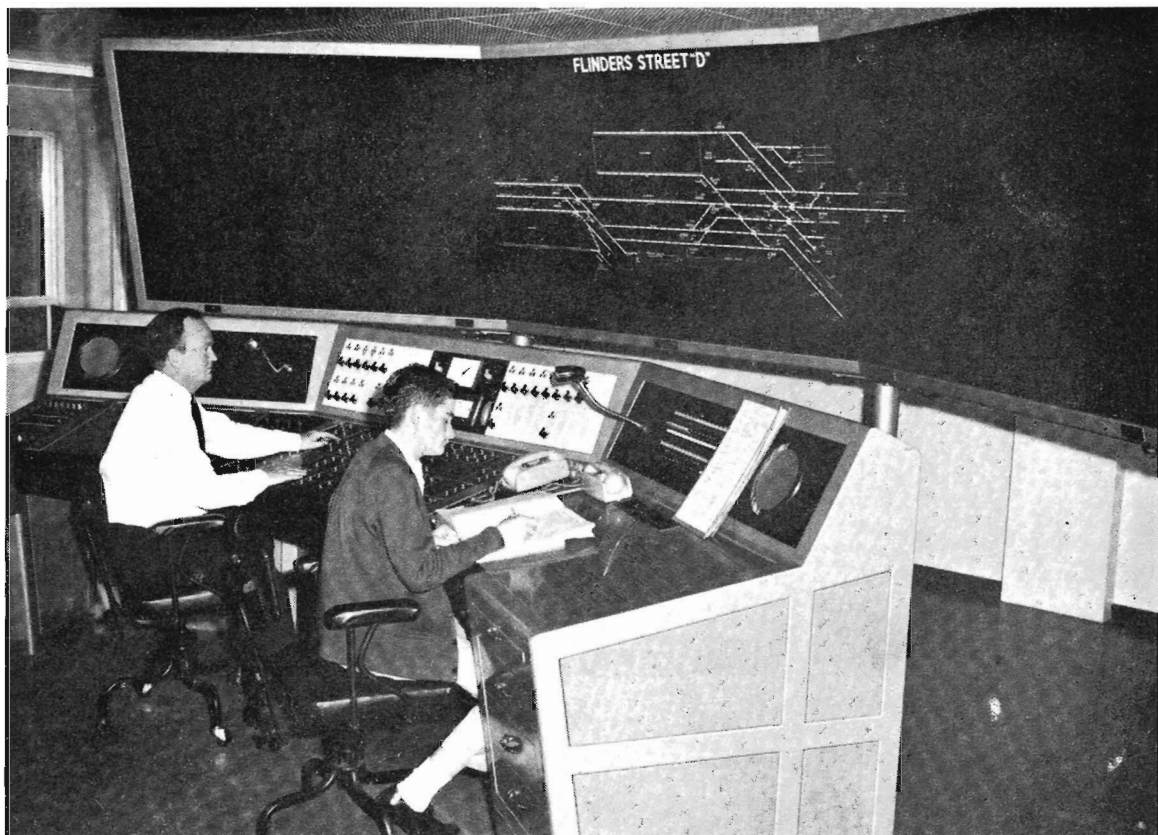
Signalman K. Kelly (left) and Block Recorder W. Grimsey at work in the new Flinders Street D Box. Space has been provided on the diagram for future requirements.
