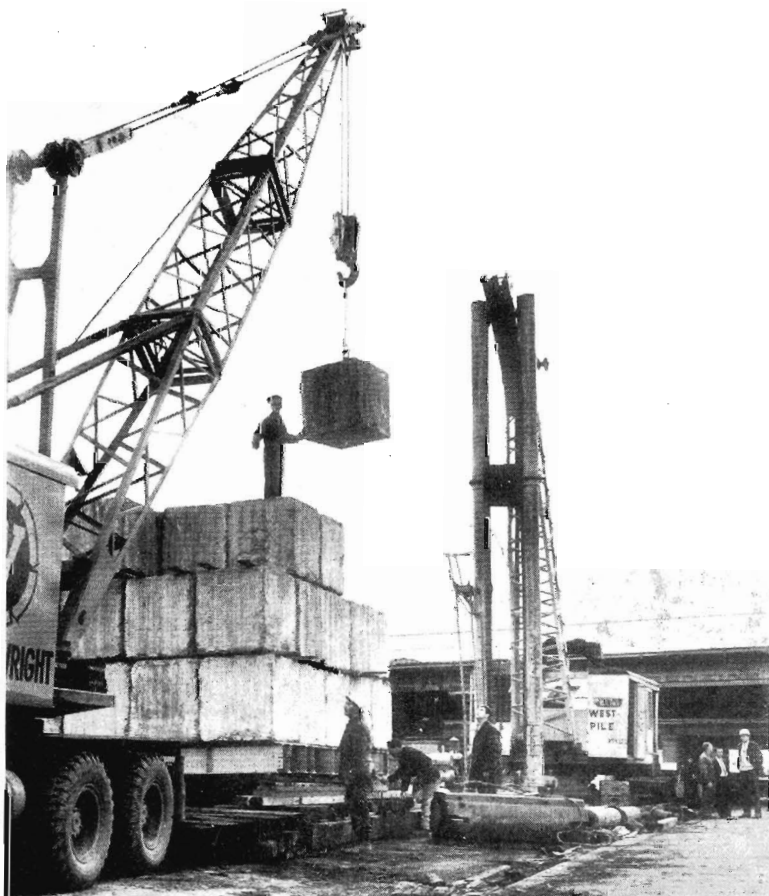
Testing piles for the new bridges across Dudley Street. To check that the piles are satisfactory and capable of standing up to requirements, a test load is applied to the pile, and its subsidence on loading, and restoration on unloading are measured. The pile shown is being loaded with a total weight of 180 tons. To the right of the test load is the pile driving frame used by the contractor to drive the pile shells.
