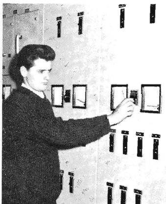
On the power supply switchboard, Apprentice Electrical Fitter I. Barnes tests D.C. supply for earth.
